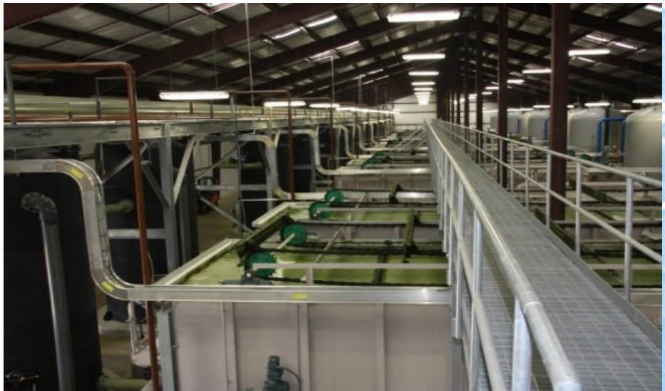
Algae Removal Process by Dissolved Air Flotation Units. Photo Credit: City of West Monroe
