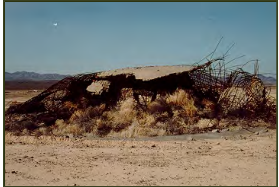
Effect of the test on the concrete shelter dome
